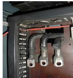
Below: Close up of burst Firetrace tube
