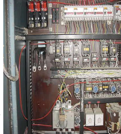
Above: Minimal damage to panel
